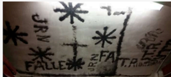
Illustration 8. Candle smoke marks on the ceiling of the basement at the BMI, Ballarat.
